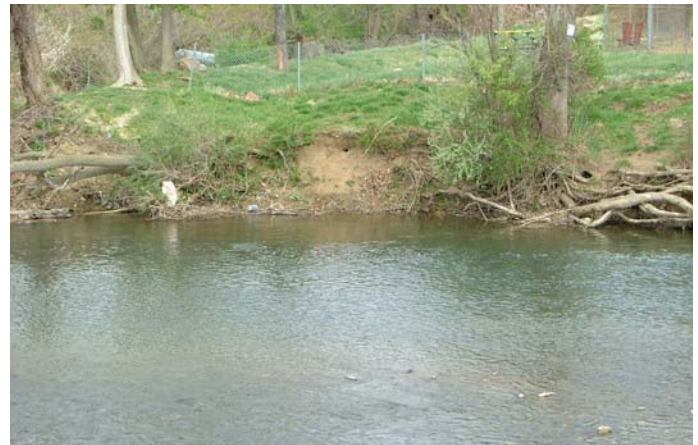
Photograph shows riverbank conditions before stabilization.
