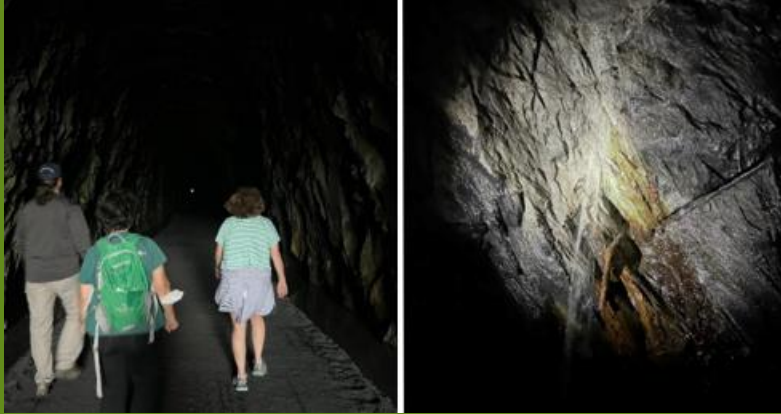
Left: Darkness in the tunnel with a distant light; Right: Trickle of water down the inner wall
