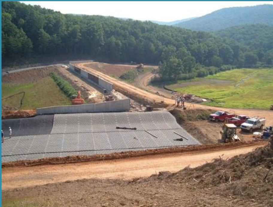
RXFIRE was hired by Headwaters Soil and Water Conservation District to clear, reseed, and cover the Stoney Creek abutment with biodegradable erosion control netting for dam safety. (Picture credit)
